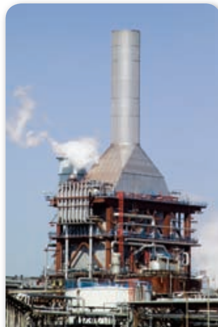
■ Figure 25.14 This cogeneration power station helps reduce energy use at an oil refinery and chemical plant in Hampshire, UK.
